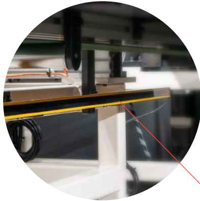
safety light curtains
